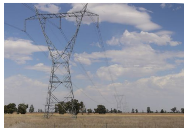
Transmission Lines and Stanchions
