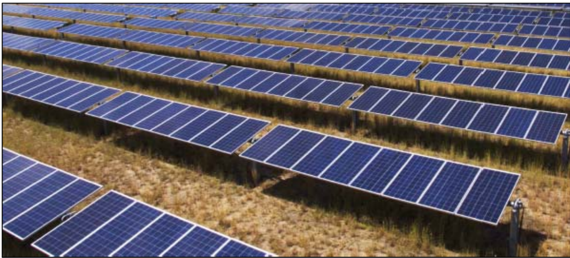
Figure 3-11 Single axis tracking system solar array
