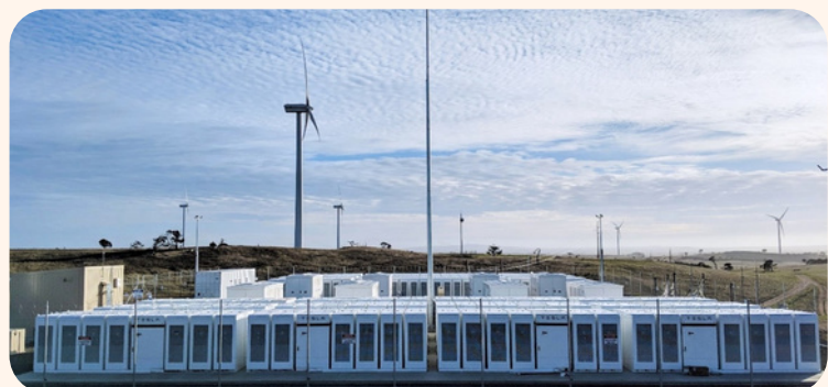
Figure 2. Lake Bonney Battery in South Australia
